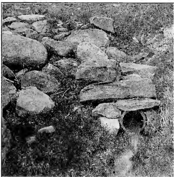
FIG. 95. A well-constructed outlet for a line of drain tile.
